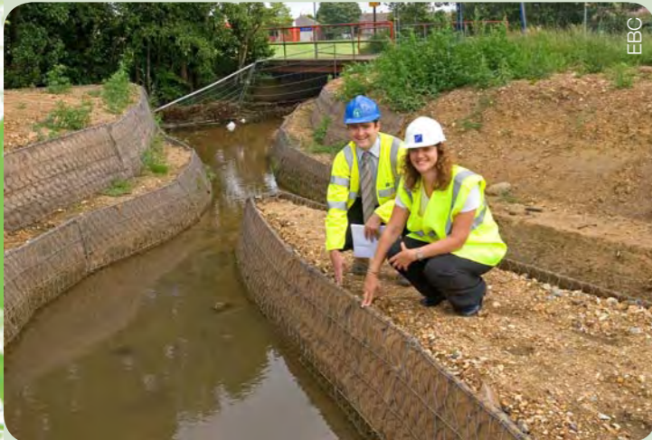
Inspecting the new channel. Plants should readily colonise the artificial matting used to shape the banks
